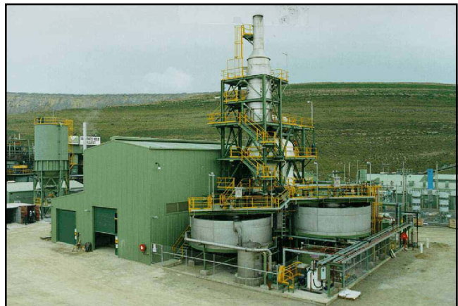
Figure 3. Discharge system and autoclave building.
